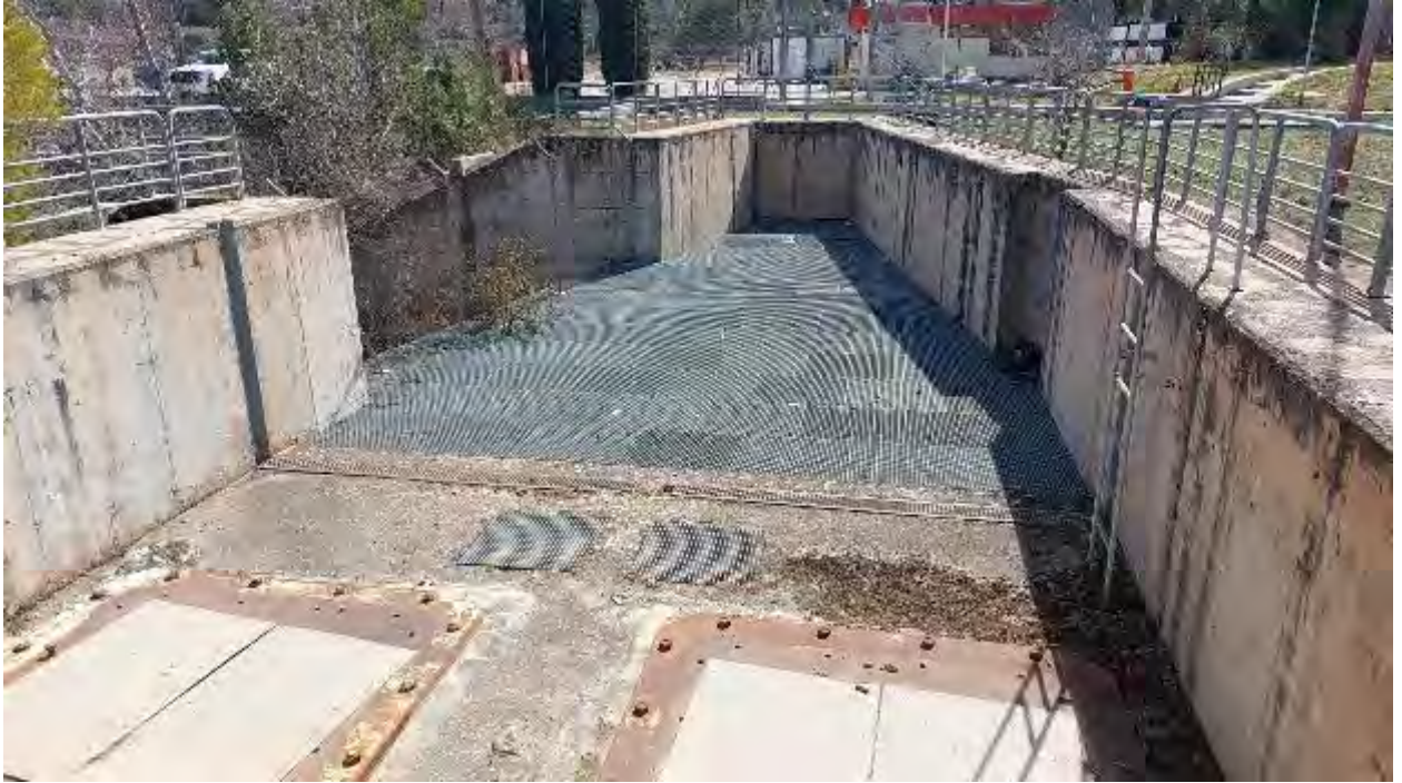
Figura 17 – Vista General Cántara Bombas 2
